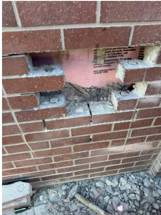
Photo 2 : Probe 1, missing through wall flashing and with cavity filled solid with grout above weep hole.
