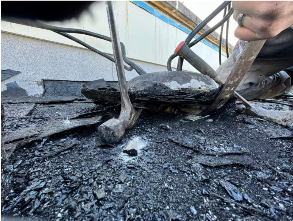
Photo 13 : Probe 4, no flashing found.
