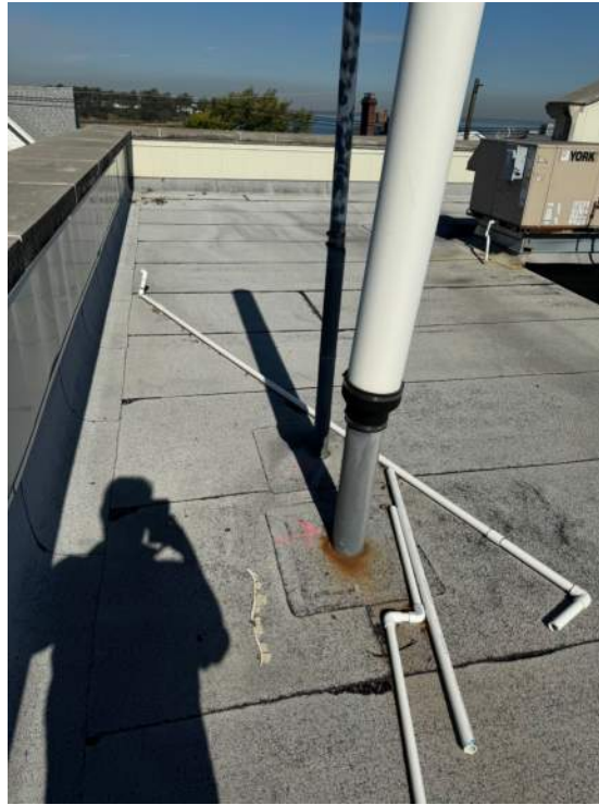
Photo 21 : Inadaquate and missing flashing components found
