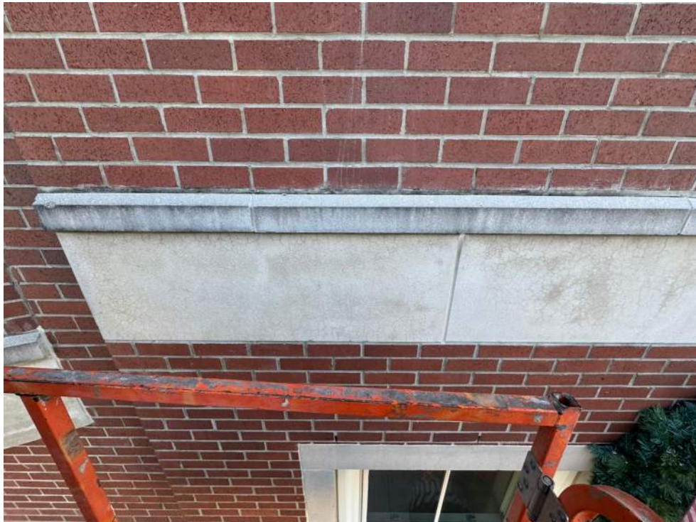
Photo 4 : Missing flashing and weeps holes at material transitions
