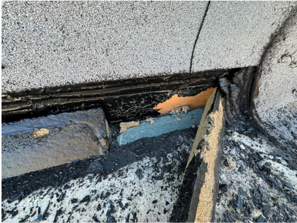
Photo 17 : Probe 7 with dry cant strip found.
