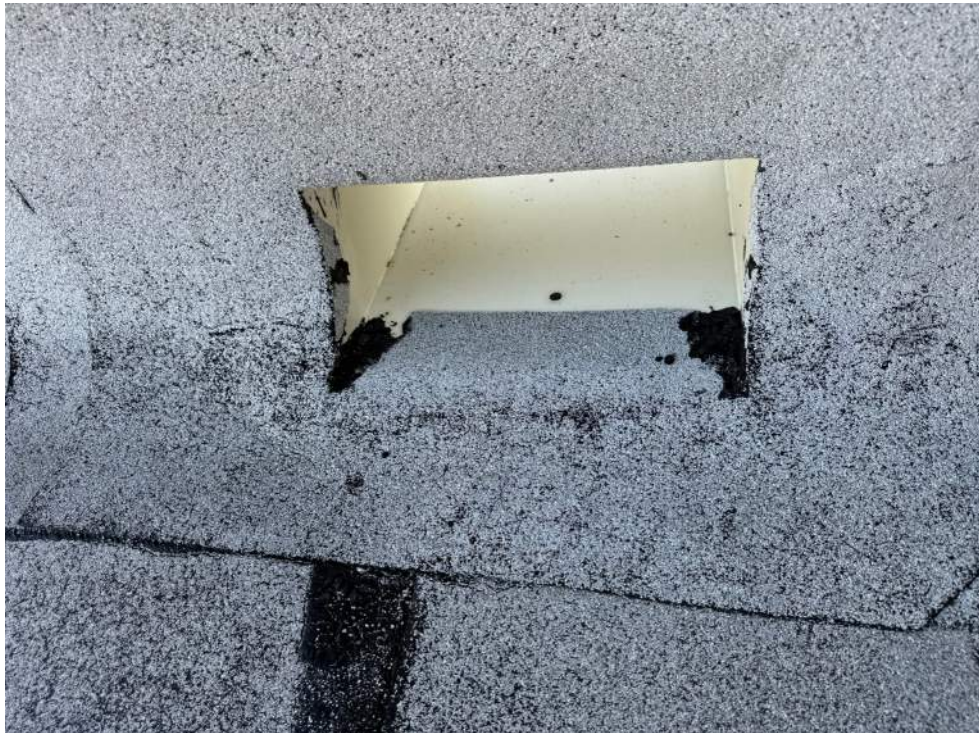
Photo 20 : Inadaquate and missing flashing components found
