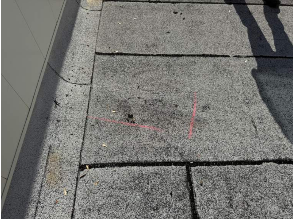
Photo 23 : Delaminating membrane found.
