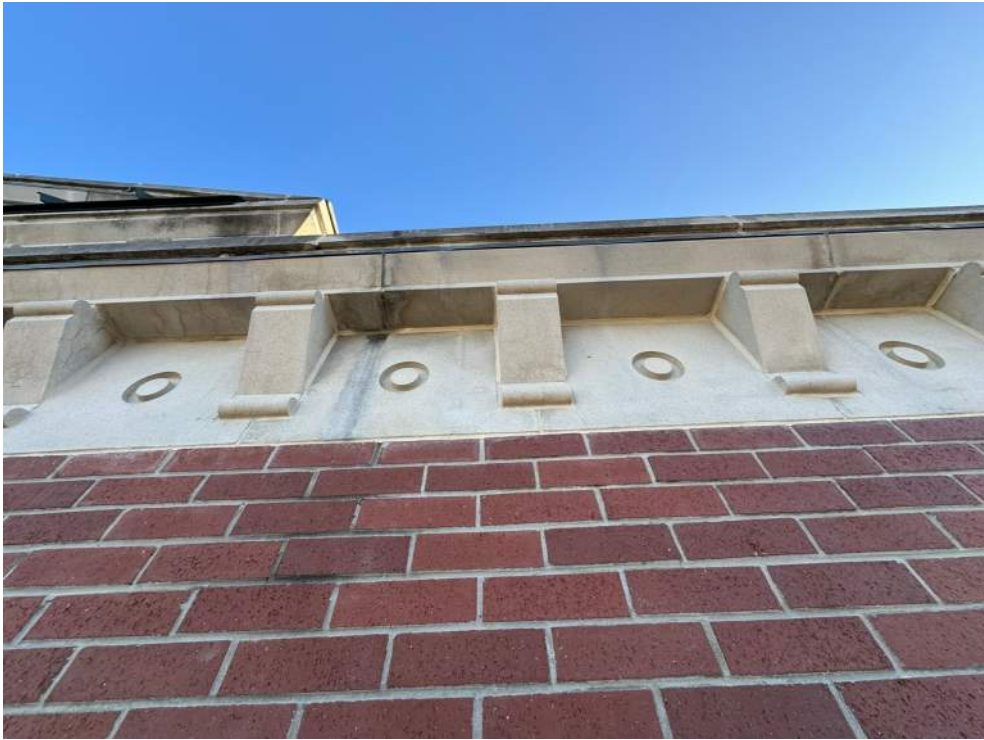
Photo 5 : Missing flashing and weeps holes at material transitions
