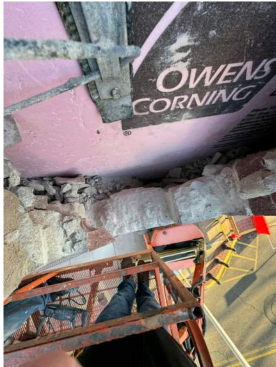
Photo 8 : Probe 2, no flashings or weep holes found looking down cavity to window head.
