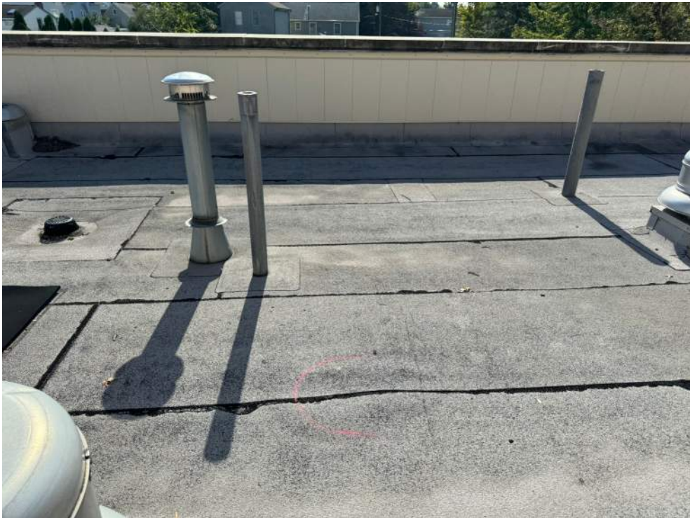
Photo 24 : Delaminating membrane found.
