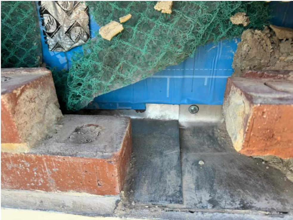
Photo 14 : Probe 5, grout filled cavity and improperly lapped flashing found.
