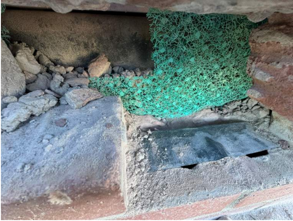
Photo 11 : Probe 3, inverted and inadequate flashing found.
