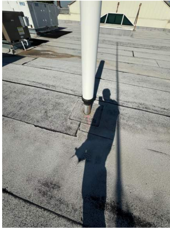
Photo 19 : Inadaquate and missing flashing components found
